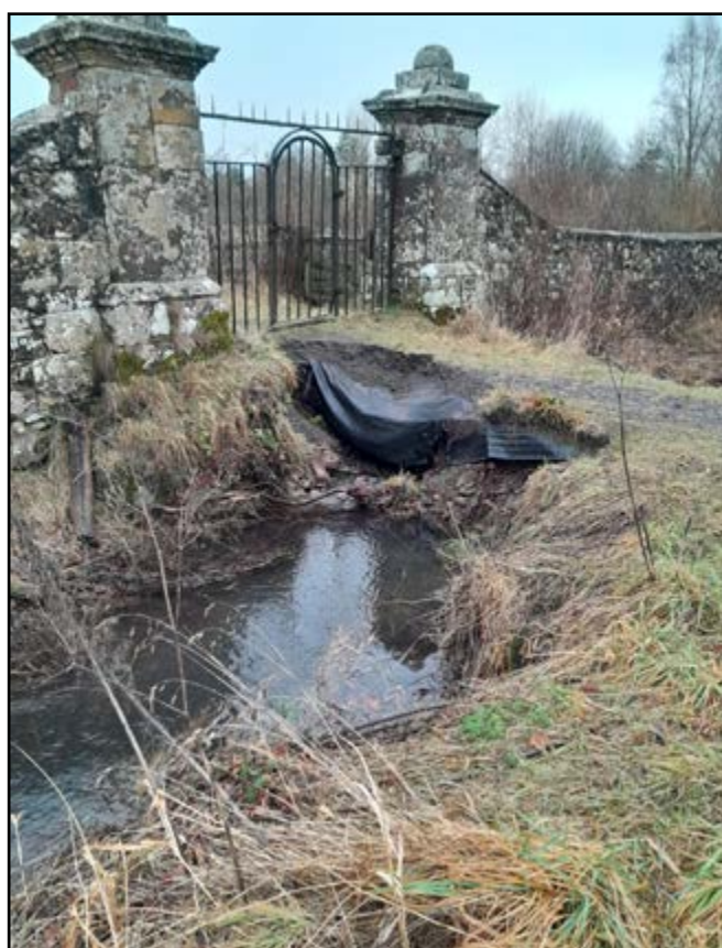
Damage at St Mary's Gate
