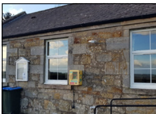
Top to bottom: Original windows with signs of rot; first window replaced; the new windows in place
