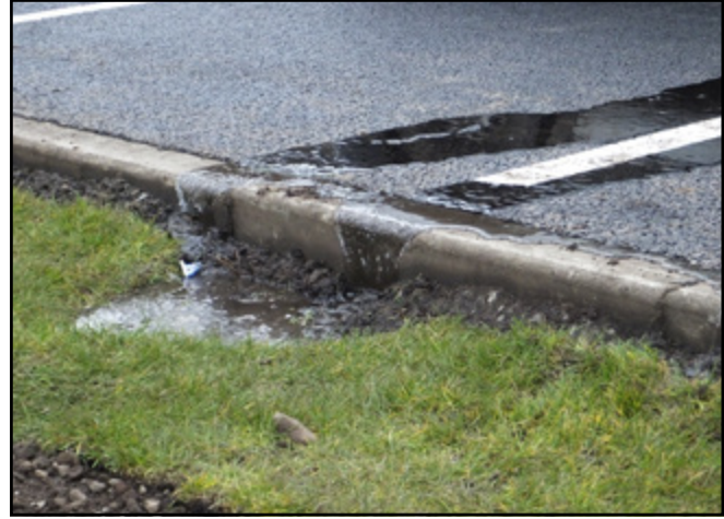
Testing: water dropped across the car park does run across and down into the raingardens
